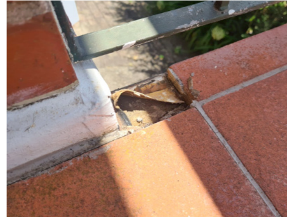
Asbestos under the tile (as a moisture barrier)
