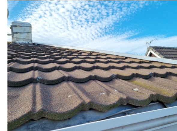
'Decramastic' metal pressed tile The bitumen layer is asbestos
