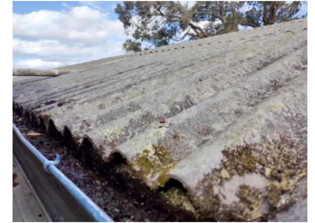
Super six roof Degradation from weathering and algae This product has reached the end of its economic life
