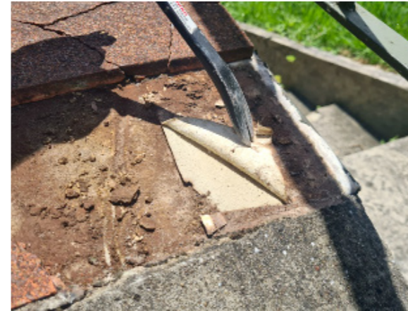
Asbestos in the paper lining under bituminous coat on a roof
