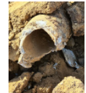
Fragment of asbestos cement pipe and buried cement pipe
