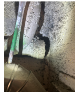
Sprayed coating overspray Overspray from asbestos coating
