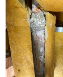
Insulation in poor condition to pipework Shows water damage to pipe and dried leak deposits in insulation
