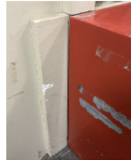
Asbestos insulating board (AIB) behind radiator unit Often used near, in or behind radiators due to its thermal insulator properties
