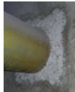
Raw asbestos used with plaster as a gap filler
