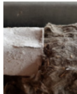
Asbestos paper wrapping to pipework
