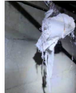
Asbestos insulation in poor condition to pipework This will likely release fibres when disturbed
