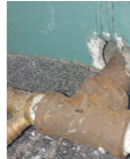
Asbestos insulating board (AIB) behind radiator unit Often used near, in or behind radiators due to its thermal insulator properties
