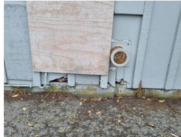
Gas heater vent sticking out of ACM board
