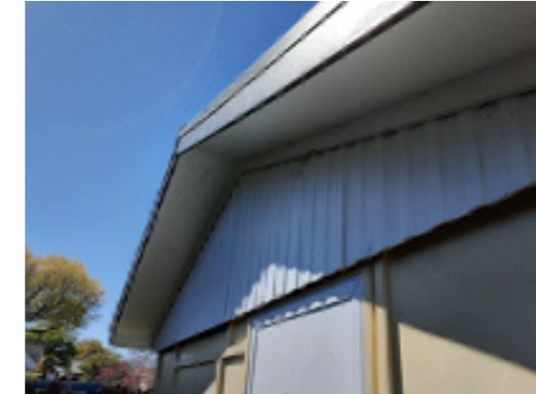
Asbestos soffit Cladding also has asbestos containing materials
