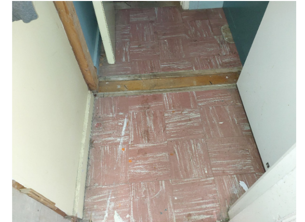
Vinyl tile flooring containing asbestos
