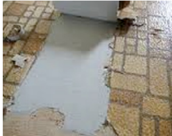
Torn vinyl flooring containing asbestos
