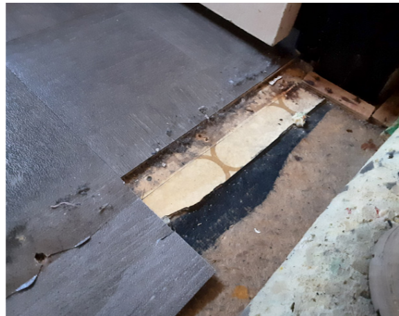
Asbestos containing materials tile plus adhesive under modern vinyl
