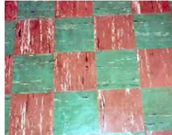
Asbestos containing vinyl tile
