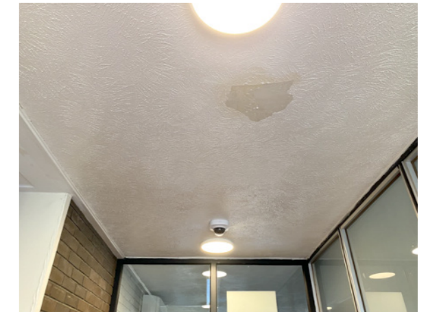
Damaged textured ceiling
