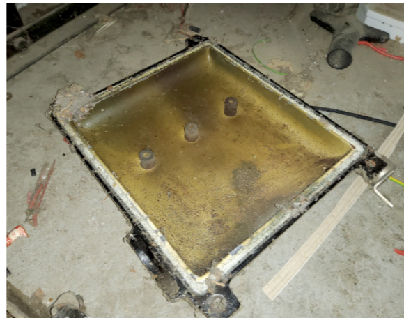
Rope seal around electrical unit door
