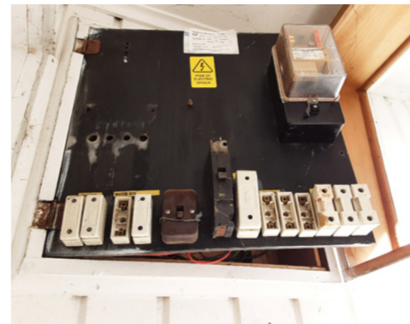
Fuse box backing board
