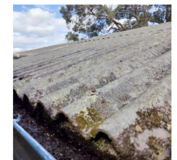
Super six roof Corrugated cement sheet containing asbestos commonly known as super 6 has asbestos in the composition. This type of product is approximately 50 years old and has reached the end of its economic life
