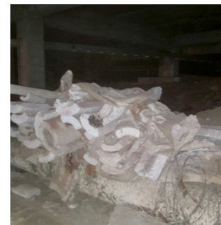
Loose lagging in basement High risk of excessive contamination
