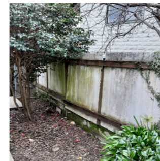
AC fencing in bad condition Common to many houses
