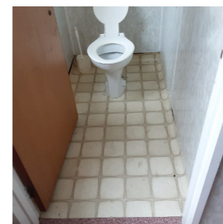
Paper backed vinyl Floor covering in bathrooms and wet area may contain asbestos in the lino or backing. The asbestos fibres in the backing can become airborne when lifted
