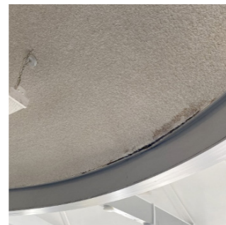
Sprayed coating on the ceiling Common to many houses
