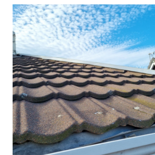
'Decramastic' metal pressed tile Pressed metal roof tiles commonly known as decramastic tiles may have asbestos in the base mastic bitumen
