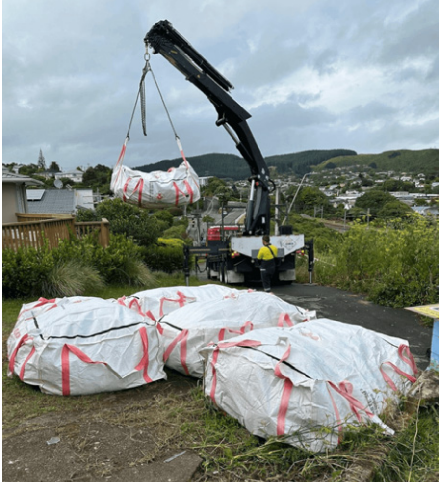
FIGURE 30: Examples of asbestos waste being removed
