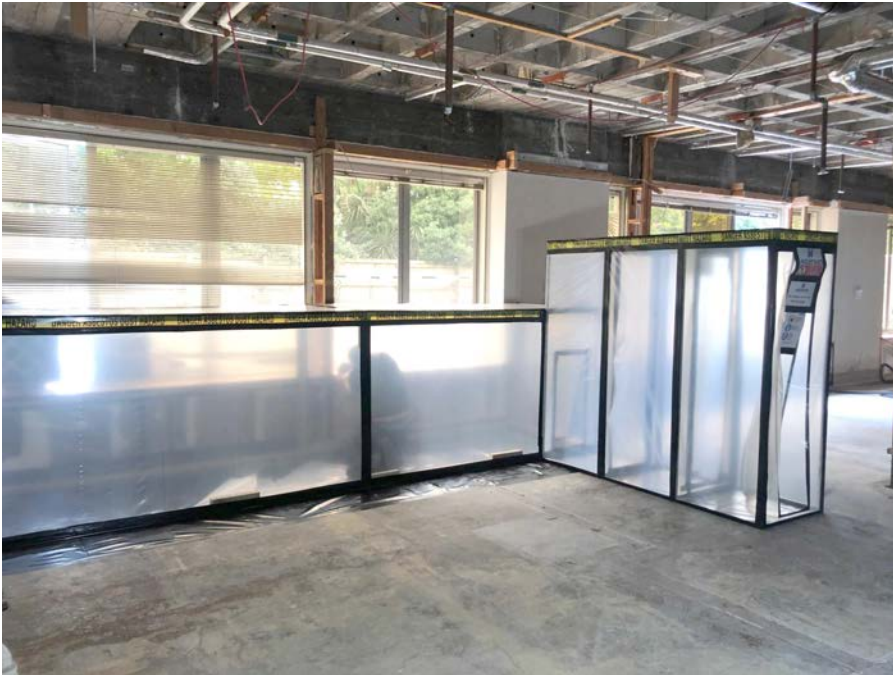
FIGURE 2: Enclosure with three-stage airlock
