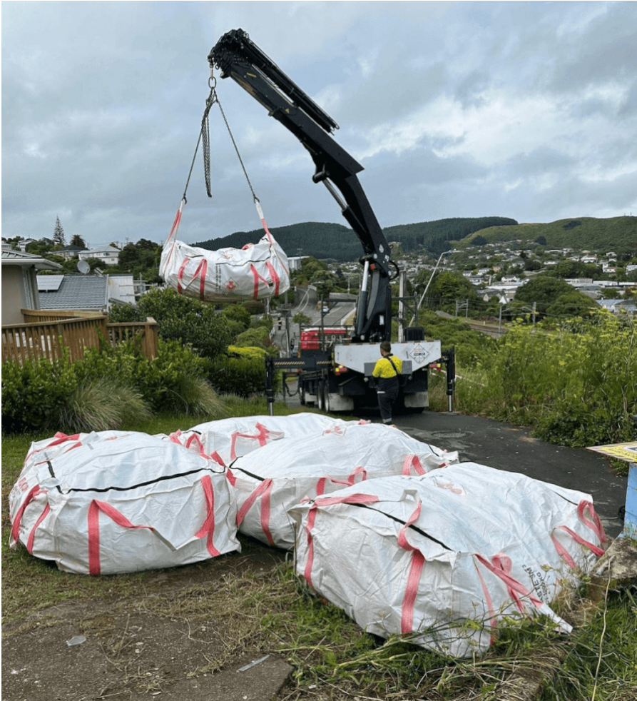
FIGURE 30: Examples of asbestos waste being removed
