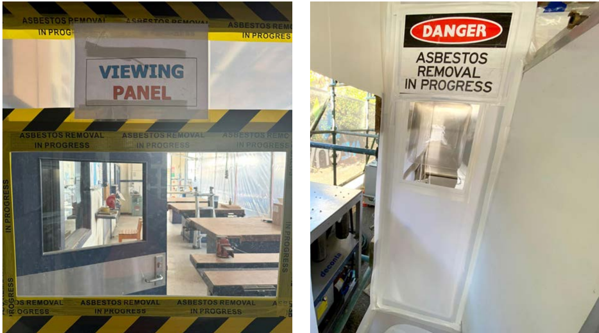
FIGURE 14: Examples of viewing panels
