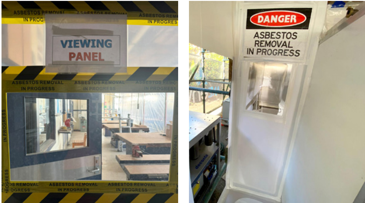
FIGURE 14: Examples of viewing panels
