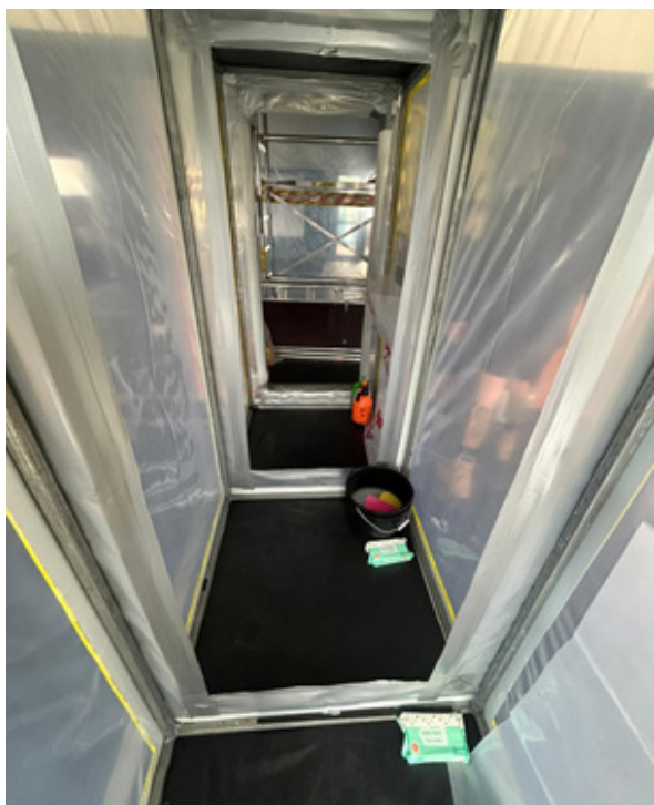
FIGURE 35: Inside view of three stage airlock with preliminary decontamination materials
