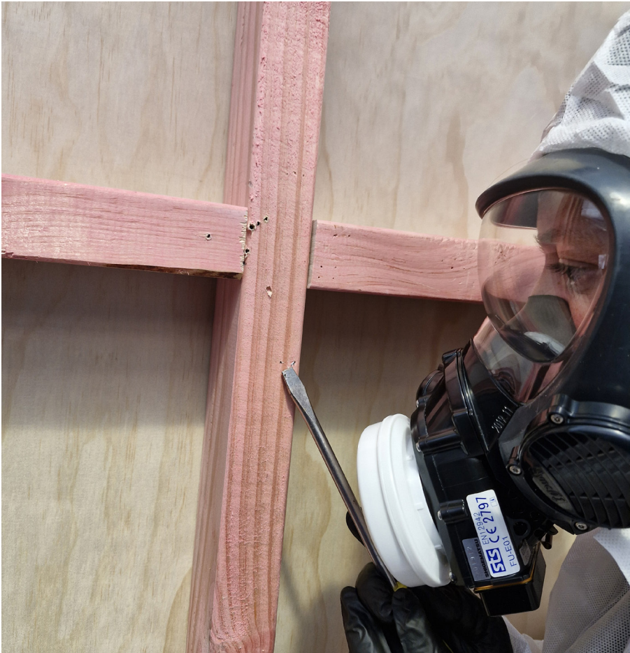
FIGURE 11: Assessor using a screwdriver to check for asbestos remnants
