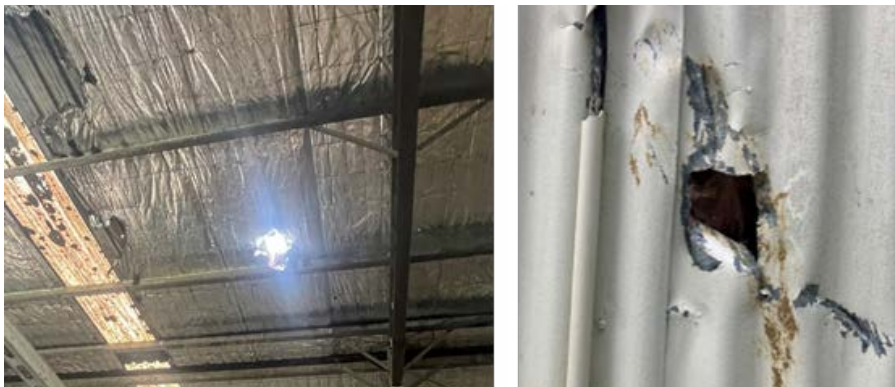
FIGURE 9: Examples of fly rock damage
