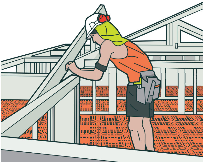
FIGURE 14: A worker installs a joist hanger from a safety deck on a residential building site
