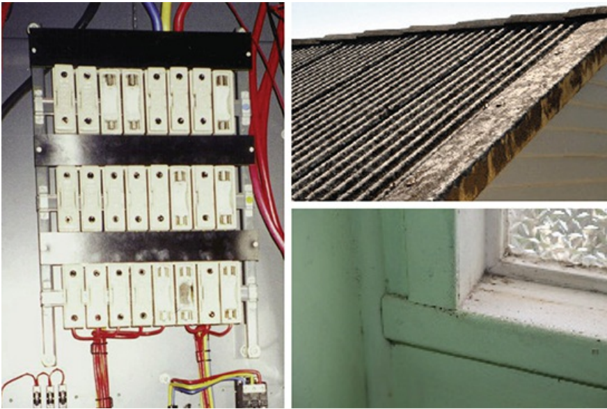
Figures 1, 2 and 3: Asbestos can be in places that you might not expect; including behind fuse boxes, in roofing, and window sills
