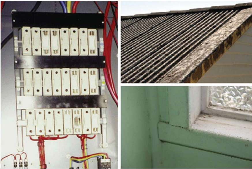
Figures 1, 2 and 3: Asbestos can be in places that you might not expect; including behind fuse boxes, in roofing, and window sills
